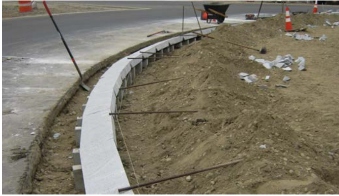
LOCATION: Route 9–Route 126/I-95 Northbound Ramps/Service Plaza Drive, West Gardiner, Maine. SOURCE: Jonathan French.
