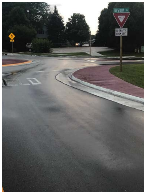
LOCATION: Bryant Road/Greenway Cross, Madison, Wisconsin. SOURCE: Ourston.
